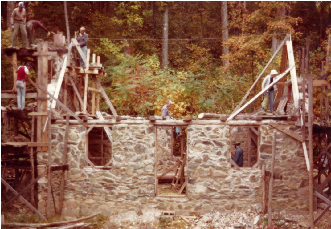
October 1981 - A 10 day work trip at the cabin and a tremendous amount accomplished - Otey Shelton atop the high scaffolding
