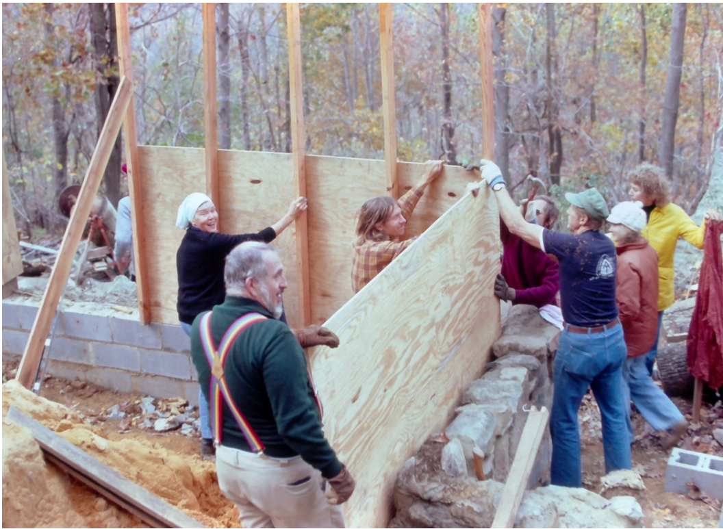
November 1979 - Foundation Work - cinderblock foundation is visible as we erect plywood - Left to Right - Margaret Crate, Gene Krah, Bob Adkisson, and Otey Shelton with hammer
