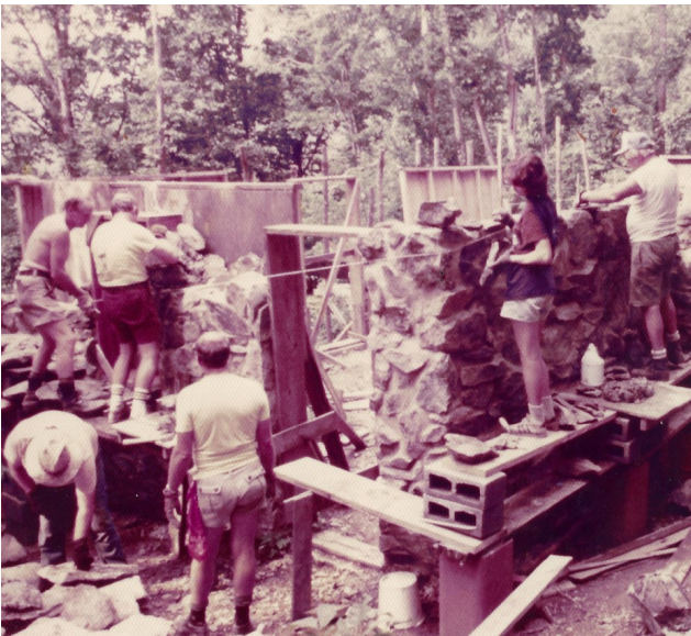
Summer of 1980 - Large Group of Workers lay rocks as the 4 cabin walls slowly rise
