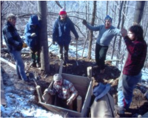
February 1979 - One of the first jobs at the cabin site - dig a hole - build an outhouse - Bill Newsom and Steve Crate - right side
